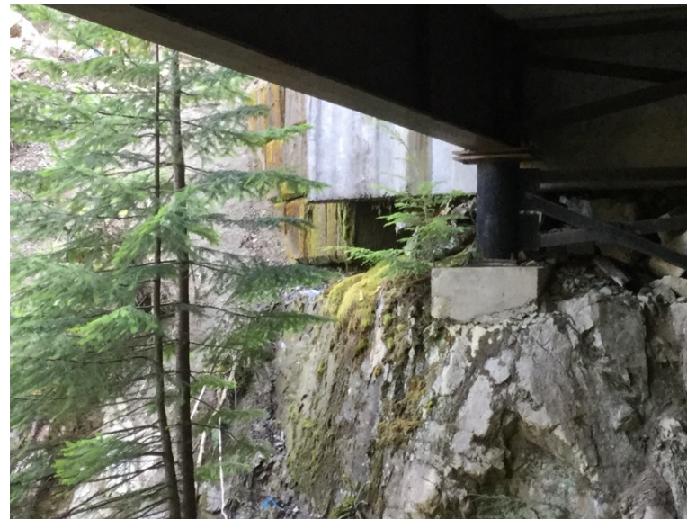
Downstream right bank wingwall undermined
